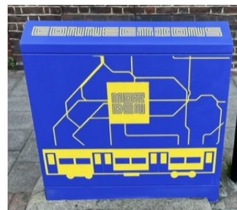
Cable box in Windermere Avenue (right)
