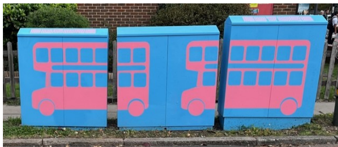
Cable box in Grasmere Avenue (left)
